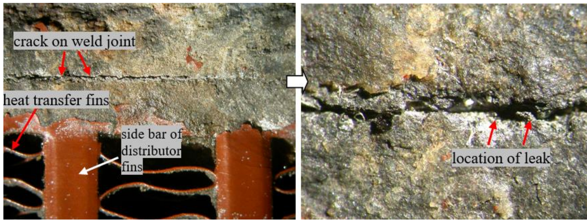
Figure 4. Close up view of the corroded surface around the weld joint of the leaked compressor after-cooler
