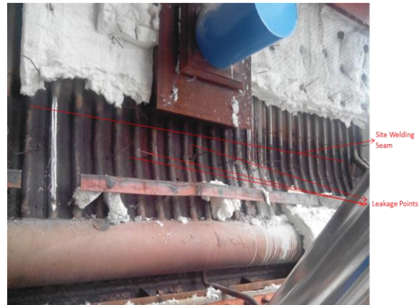
Figure 1. Photograph of cage superheater tubes after the accident showing locations of tube leakages
