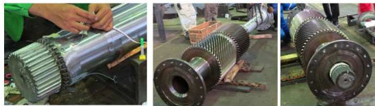
Figure 3. A new quill shaft and its installation into the pinion second reduction assembly
