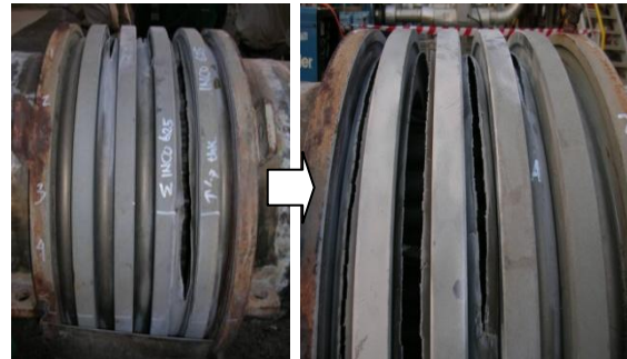
Figure 2. The ruptured expansion bellows showing four of its five bellows convolutions that were severely damaged due to cracking. Most of the cracks rupture occurred on the upper side or top side of the bellows convolutions
