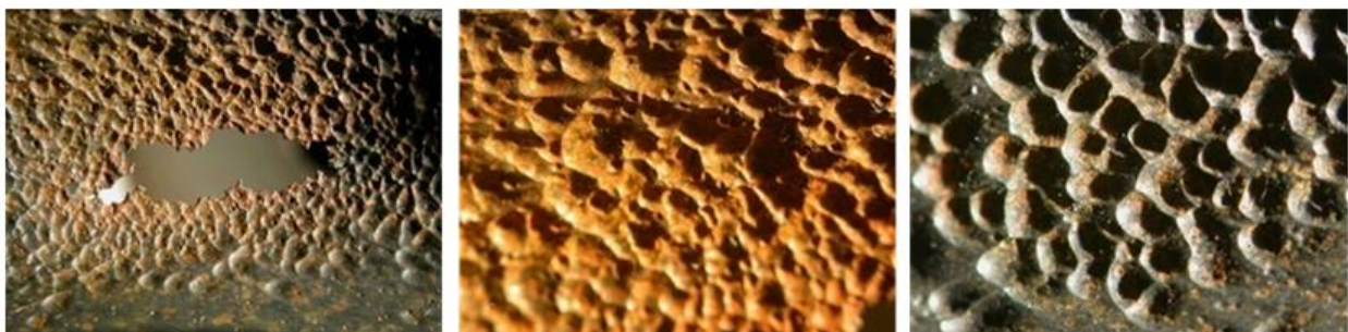
Figure 4. The inner wall of the elbow tube 1A showing a pinhole and a rough and jagged appearance in the cavitation-erosion area
