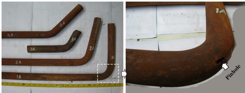
Figure 2. Four elbow tubes (1A to 4A) cut away from the low pressure evaporator evaporator outlet header, where one of the elbow tubes (1A) shows a pinhole on the outer side of the elbow curvature
