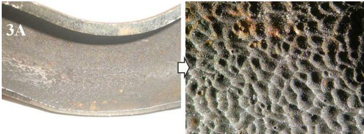
Figure 6. The damaged area due to cavitation-erosion in the elbow tube 3A showing similar rough and jagged appearance as shown in Figures 4 and 5, but at a lesser degree and no formation of any pinhole observed
