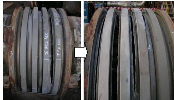
Figure 2. The ruptured expansion bellows showing four of its five bellows convolutions that were severely damaged due to cracking. Most of the cracks rupture occurred on the upper side or top side of the bellows convolutions
